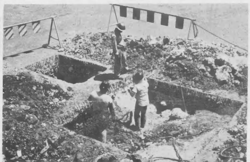
EXCAVATORS MEASURE thickness of the coral in front of Combination Units 5 through 8. The holes, some of which are shown here, will assist engineers in designing convection section additions.
